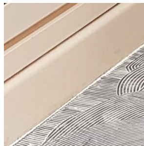
Silicone to the shower/ floor junction
